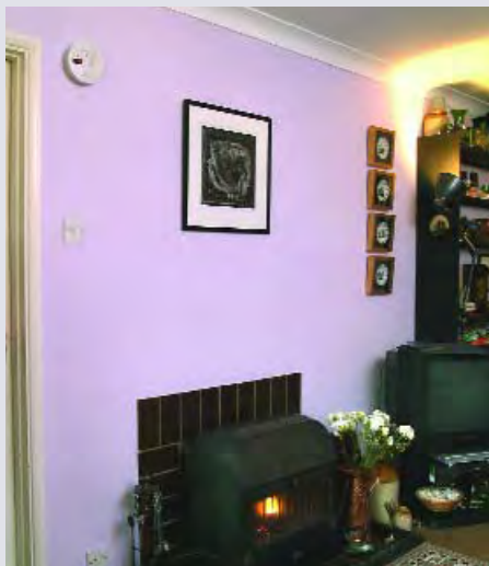
CO alarms are recognised in HHSRS as a means of working towards 'Decent Homes'.
